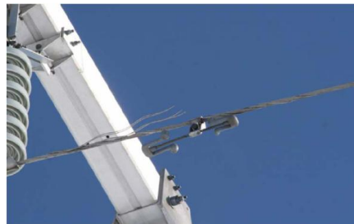
Fig. 1. Wire fracture due to Aeolian vibration.
