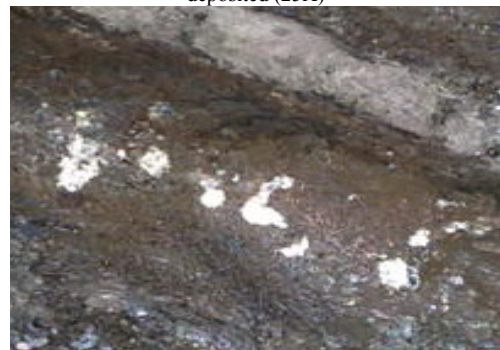
Fig 12: Absence of cracks in 15mm thick Mild Steel welded with 200°C pre-heating
