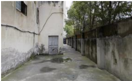
Fig. 2. The wall is falling off.
