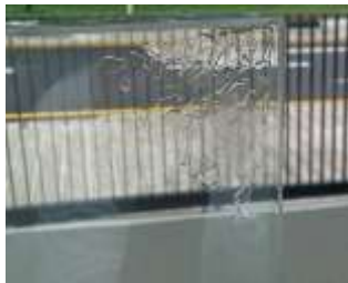
Fig. 2. Tree shape delamination.
