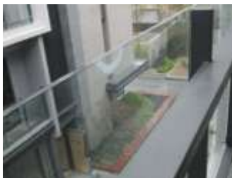
Fig. 3. Fan shape delamination with moisture.
