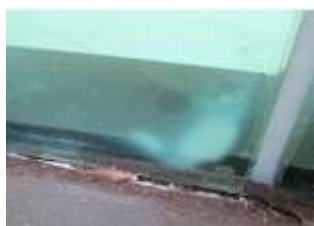
Fig. 4. Tree shape delamination with moisture.
